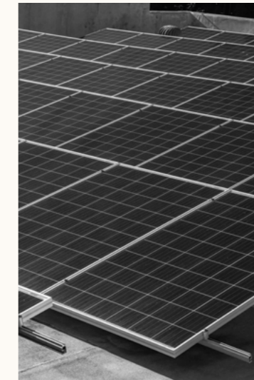
▲ Solar panel installations
